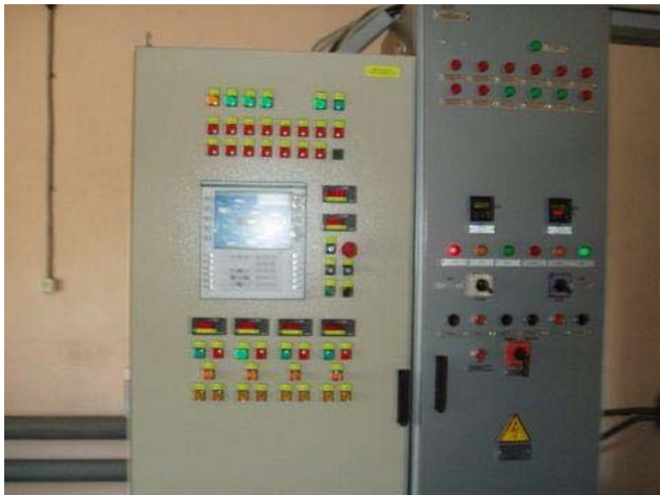
Figure 10: Boiler's automatic equipment control panel
