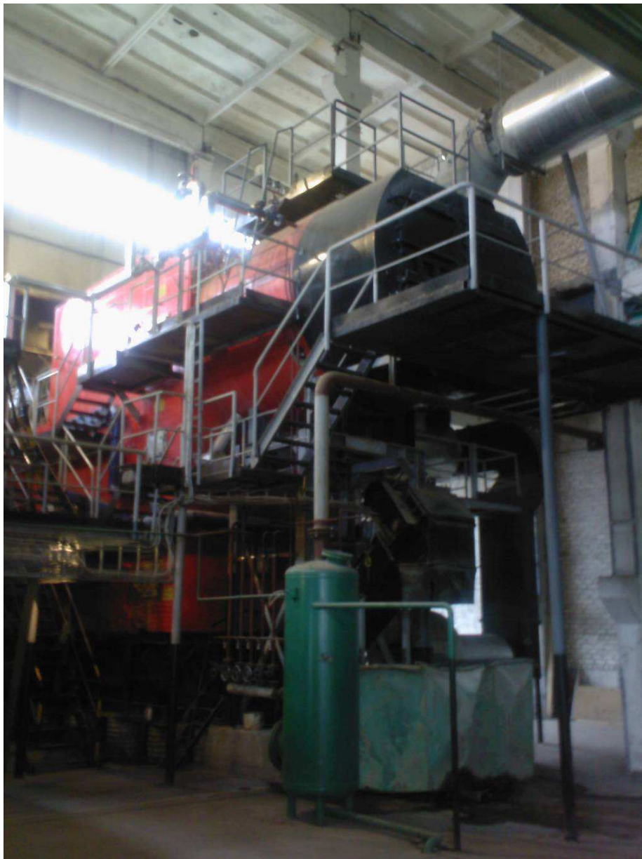
Fig. A.4-4. WEISS – Dreizugkessel Type DB-5000-OV-D boiler working on BWW
