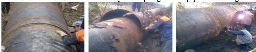
Figure 6. Application of two-layer sleeve – from left to right: adjustment of the rings and sleeve, assembling of the sleeve (rings on place), welding (a chain of several sleeves is shown which is covering multiple defects).
