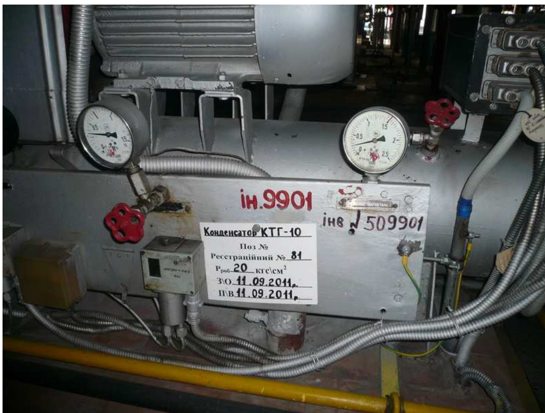
Picture 2.9. Refrigerator of cooling machine
