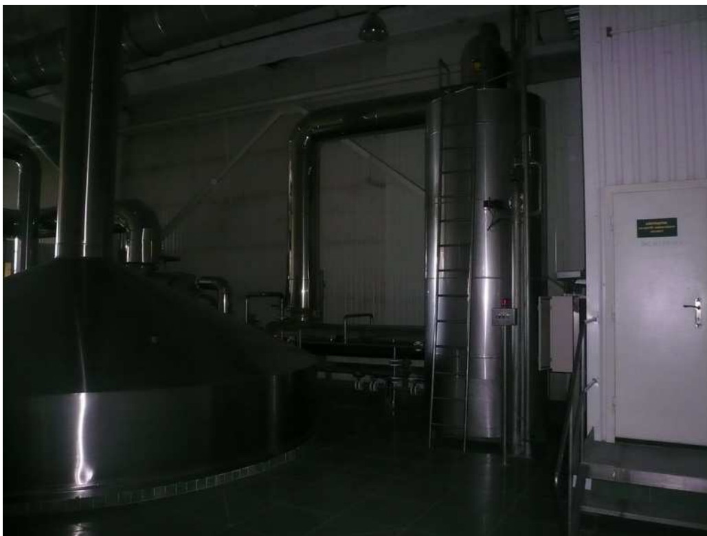
Picture 2.11. Vacuum evaporator and heat exchanger of brewing line №5
