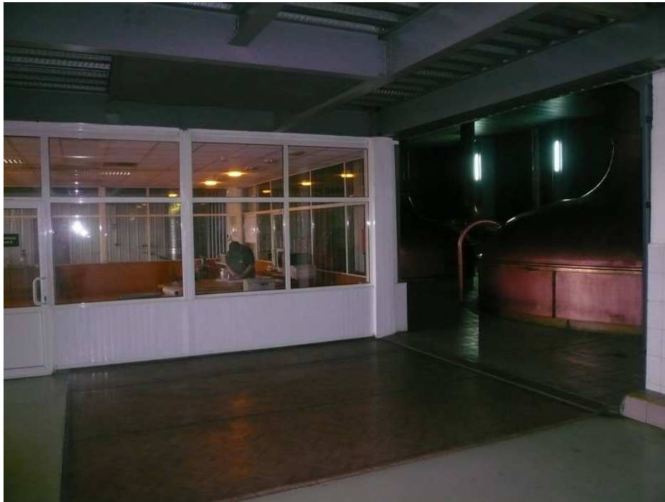
Picture 2.14. Control room of brewing lines 2 and 3
