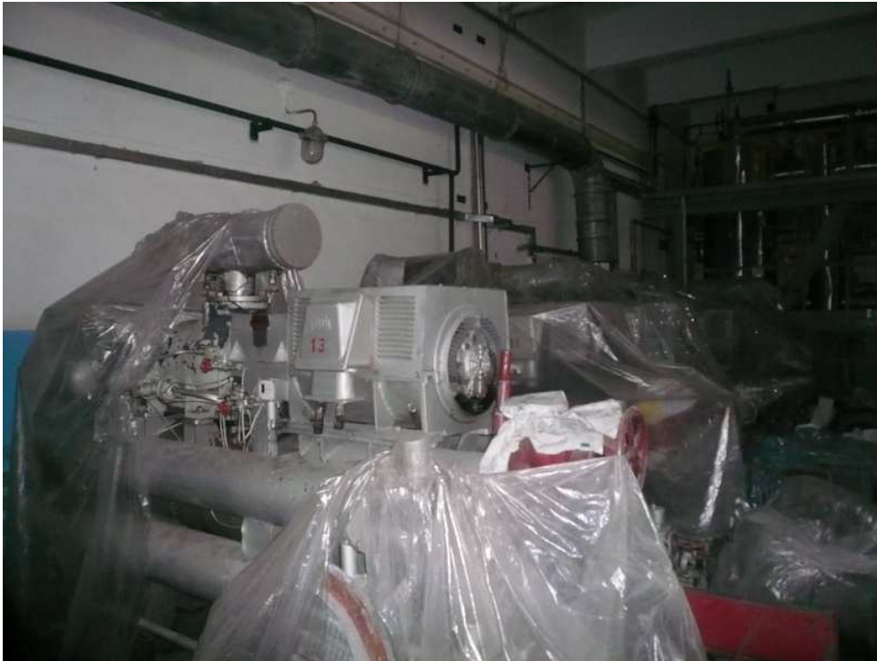
Picture 2.2. Old refrigerating machine - ammonia compressors 21A-410-7
