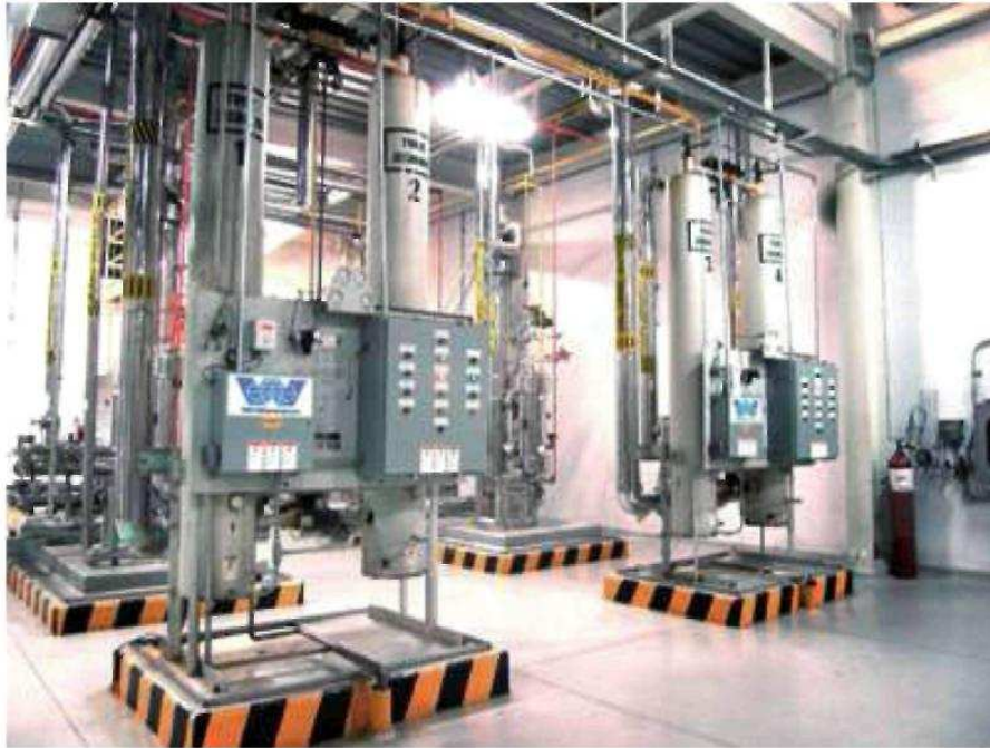
Picture 2.4. Wittmann Brewery CO2 recovery system
