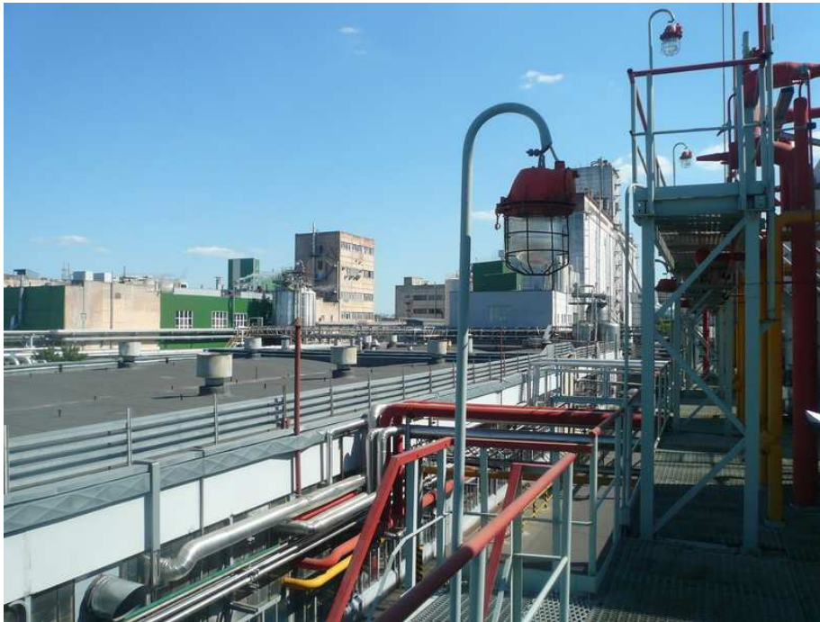
Picture 2.8. place with cooling towers, on the left there is building of refrigerating compressor shop 2007 – replacement of 2 air compressors with new, more efficient ones;
