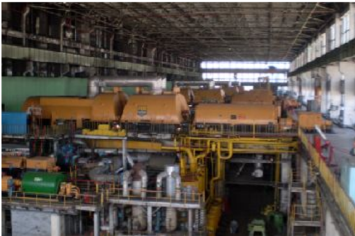
Figure 1. The Turbine Hall of the Prydniprovsk TPP
