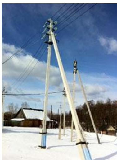
Fig.13 Towers of overhead power lines
