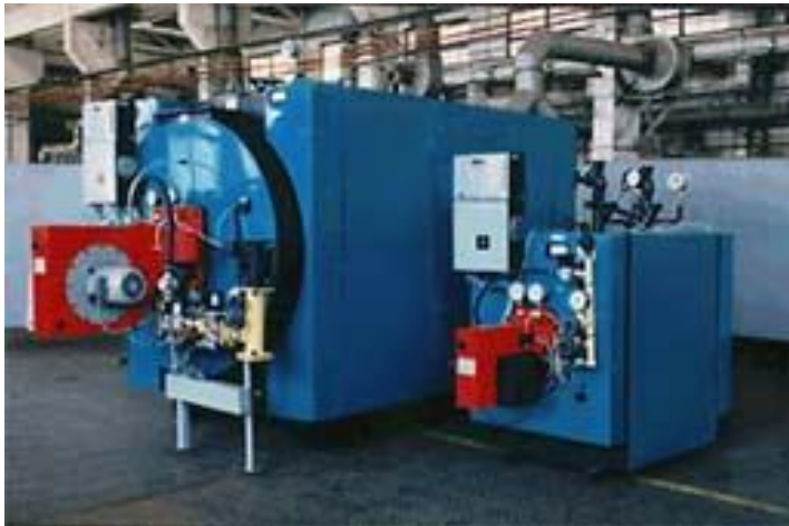
Fig.5 Boiler VK-21 with efficiency 92%.
