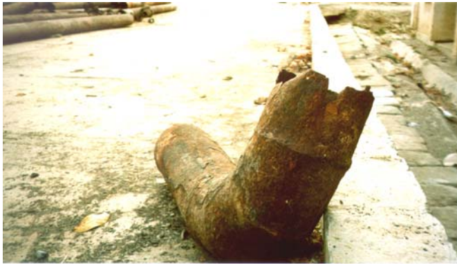
Figure 1: Existing corroded district-heating pipe from Tasca.
