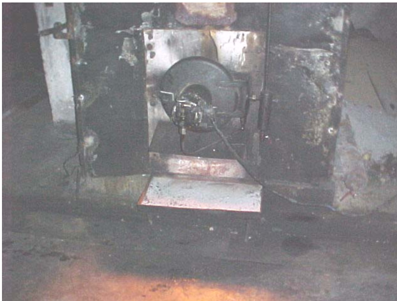
Fig. 3: The existing boiler in Gheorgheni. Who will dare to predict the efficiency
