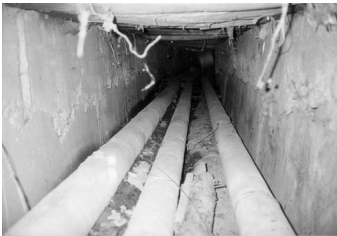
Figure 2: Looking into a concrete pipe channel in Tasca containing earlier insulated district heating pipes
