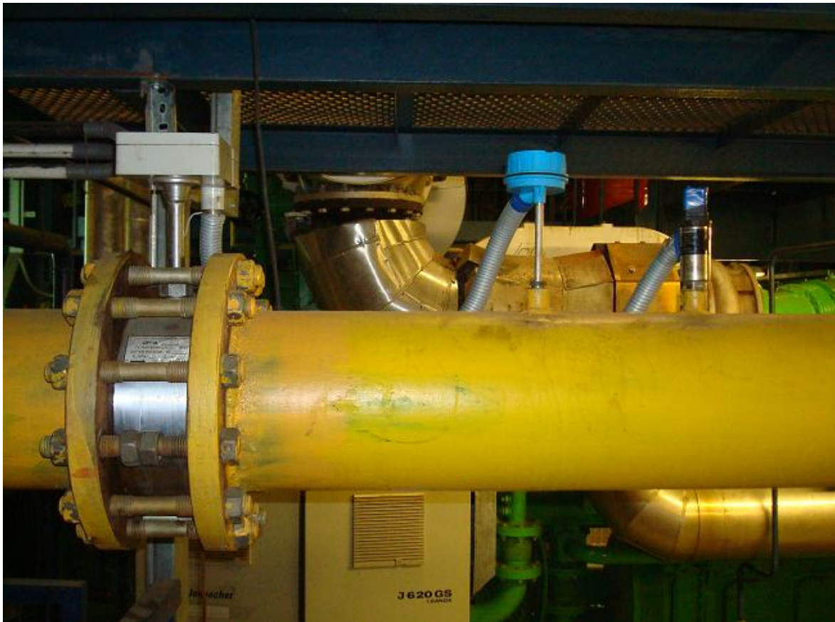
Figure 5: Gas flow meter DRG.M-10000 12 temperature sensor Metran 274-02 and pressure sensor Vegabar-14 of metering system for gas record BKT.M at fuel gas pipeline of CHP unit.
