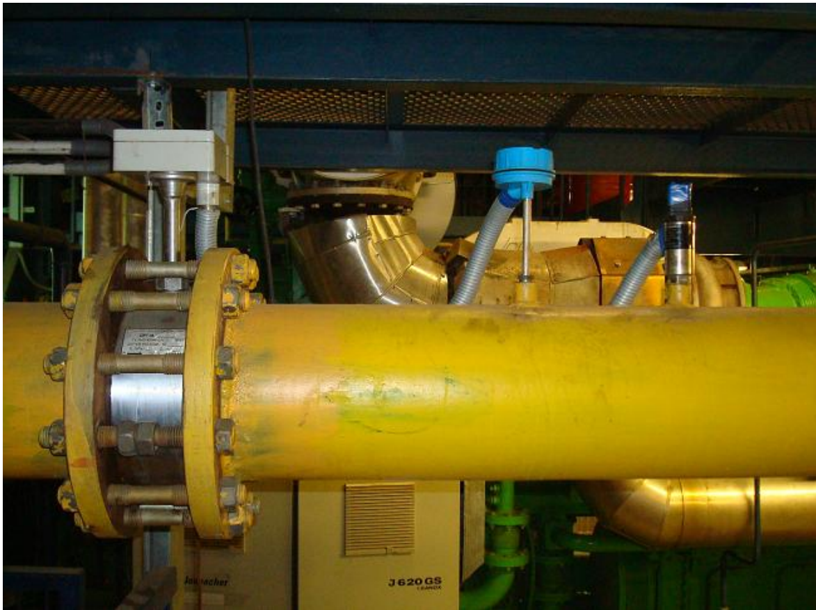
Figure 5: Gas flow meter DRG.M-10000 10 , temperature sensor Metran 274-02 and pressure sensor Vegabar-14 of metering system for gas record BKT.M at fuel gas pipeline of CHP unit.
