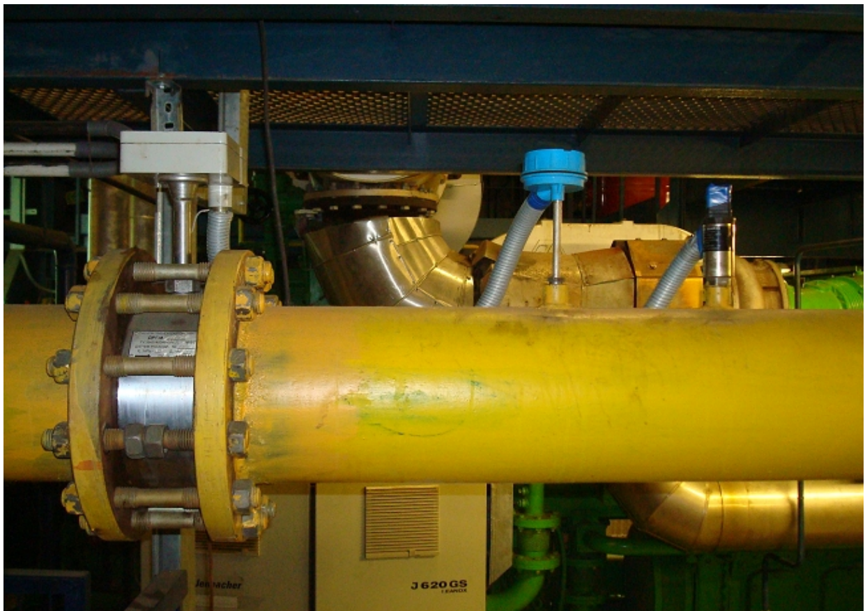
Figure 5: Gas flow meter DRG.M-10000 14 temperature sensor Metran 274-02 and pressure sensor Vegabar-14 of metering system for gas record BKT.M at fuel gas pipeline of SS CHP unit.
