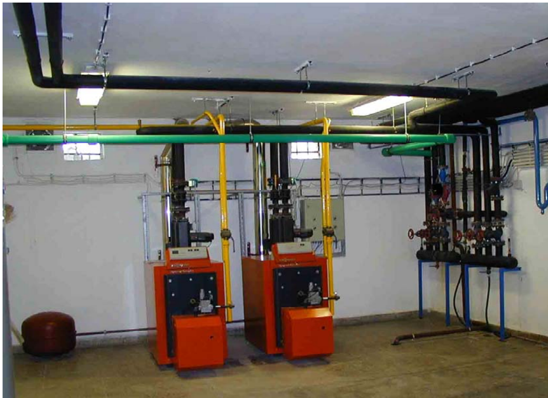
Figure 3: Gas boiler for hot water production
