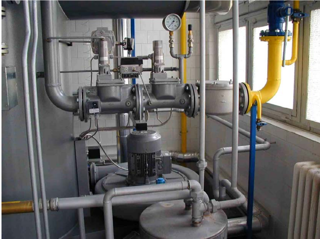
Figure 4: Gas steam boiler for steam production
