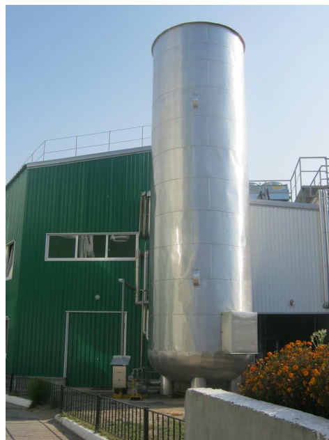
Рис.10 Heat exchanger for disposal of evaporation of boiler deaerator
