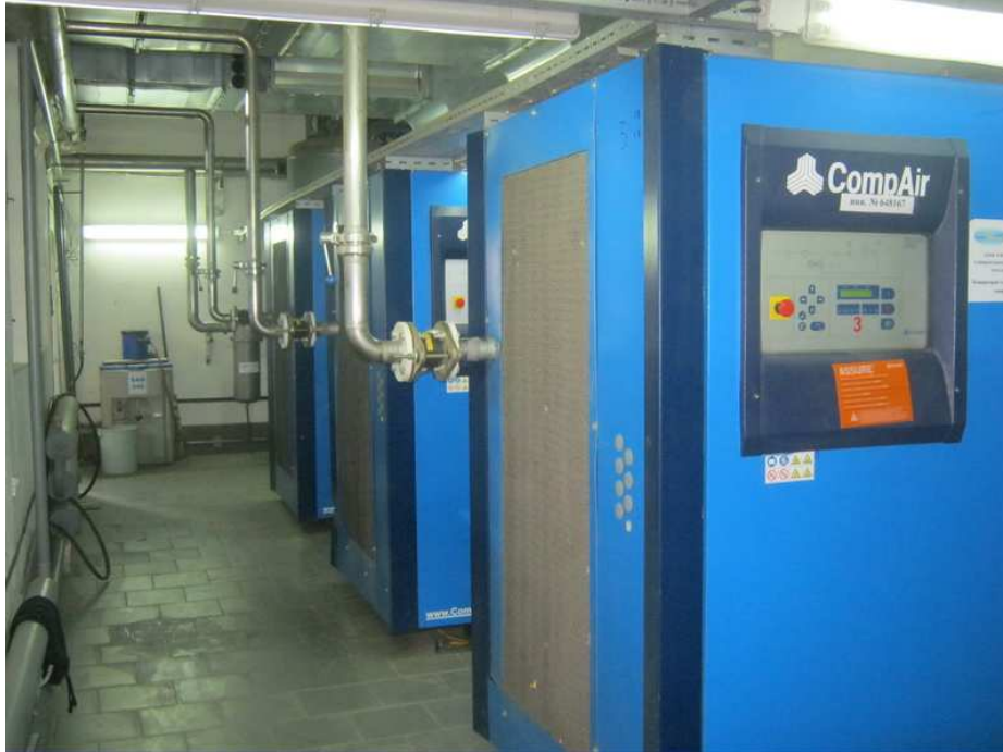
Figure 5 Air compressors Comp Air L132-7,5 – 3 units.
