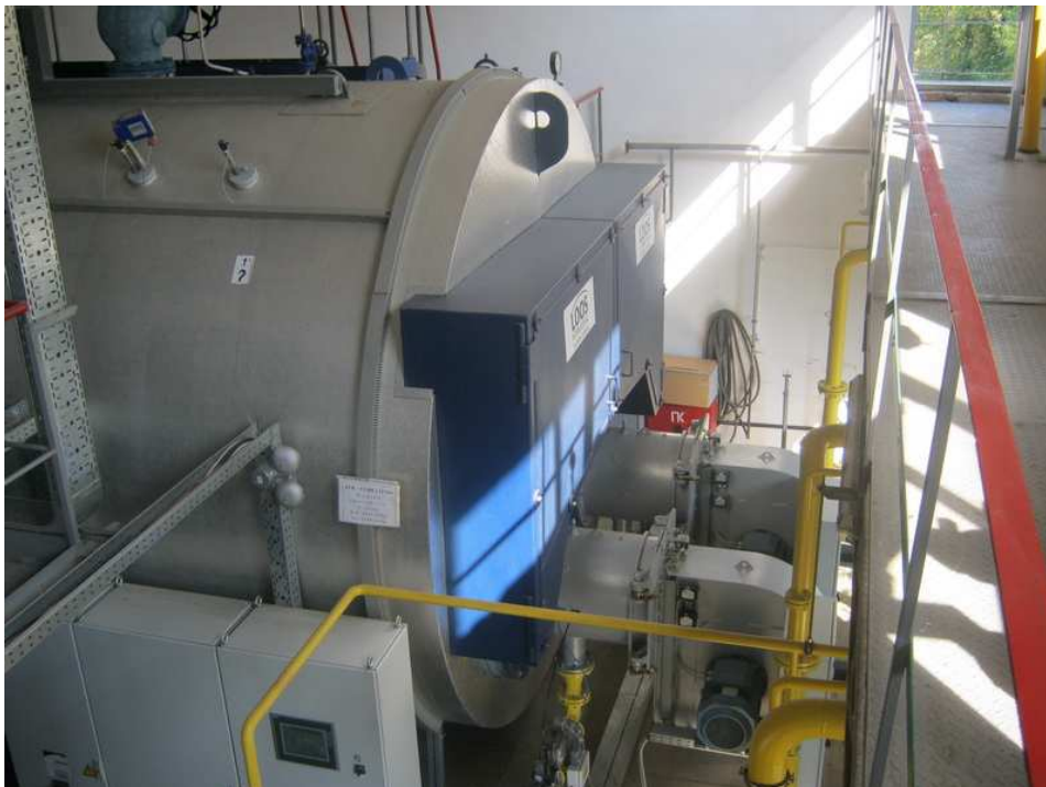
Figure 4 Boiler LOOS int ZFR-23000
