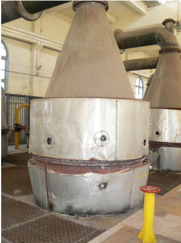
Figure 3 Single reactor from Neochim nitric acid plant
