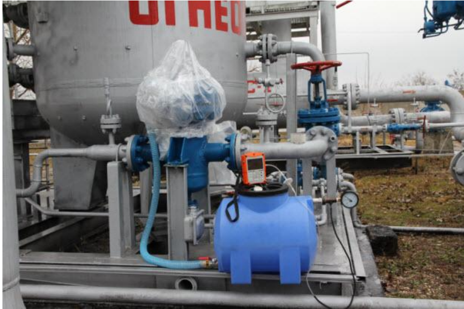
Figure 3. Photo of the installation for the quantitative measurement of methane leaks.
