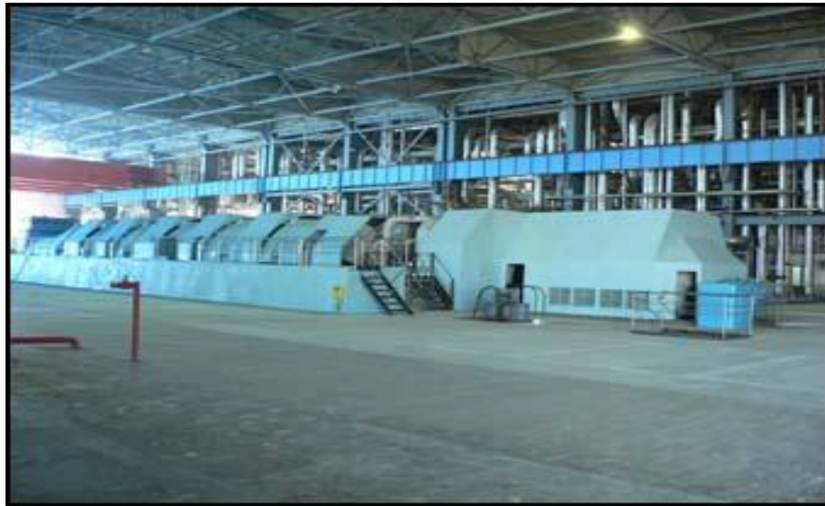
Figure A.4.2.2 – A photo of K-800-240-5LZM turbine
