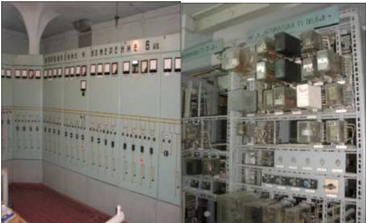
Figure 9. The Control Panel of the Substation before and after the Reconstruction
