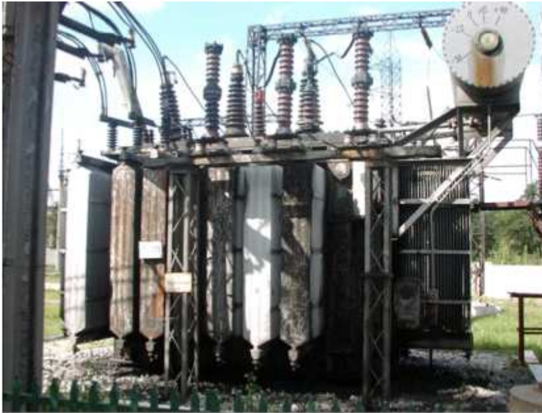
Figure 6. The Power transformer at the Substation before the reconstruction
