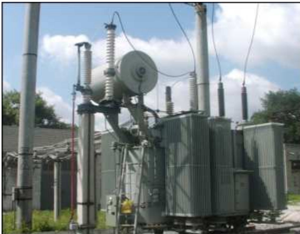
Figure 7. The The Power transformer at the Substation after the reconstruction
