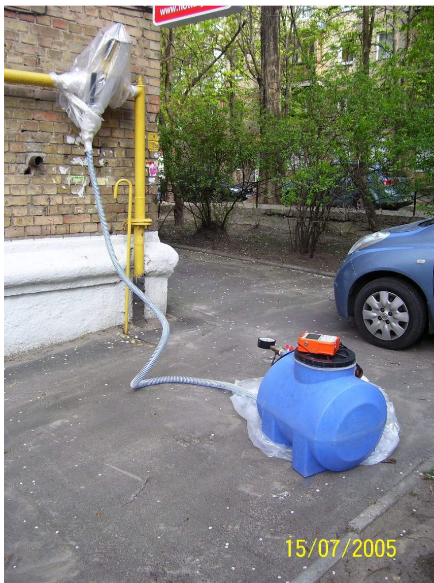
Pic. 3. Photo of a plant for quantitative measurement of methane leakage
