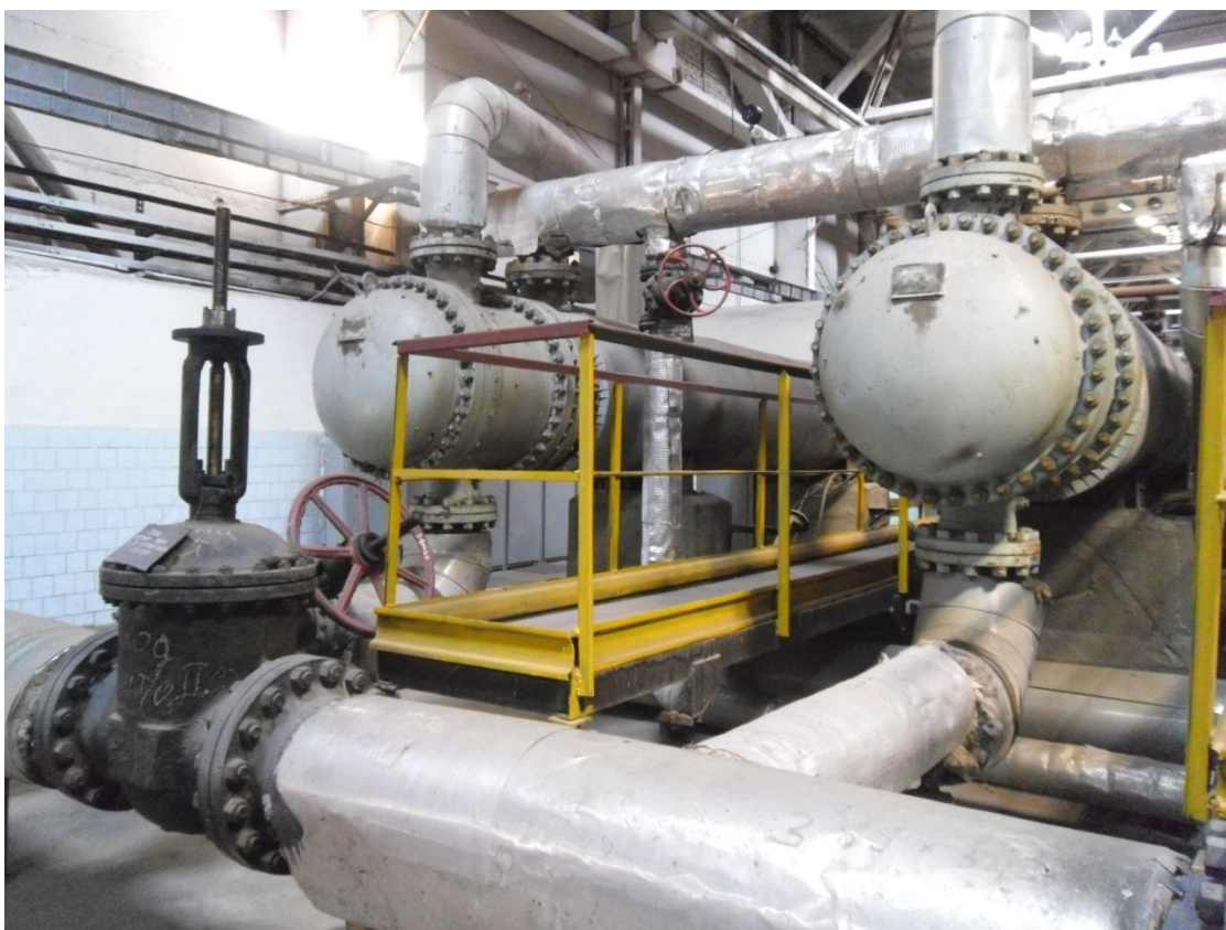
Figure 10 – Waste heat utilization unit at the site of heavy tyres production
