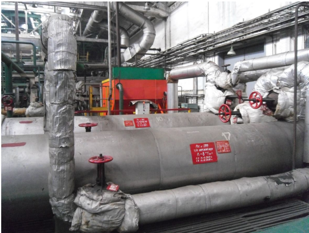
Figure 3 – Waste heat utilization unit at the main production site
