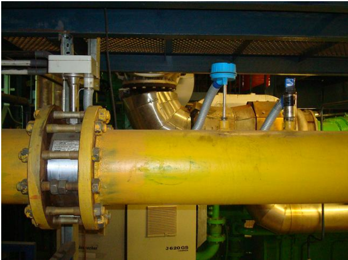
Figure 5: Gas flow meter DRG.M-10000 13 , temperature sensor Metran 274-02 and pressure sensor Vegabar-14 of metering system for gas record BKT.M at fuel gas pipeline of CHP unit.
