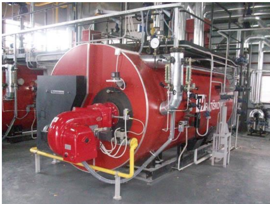
Figure 4 - General view of furnace boiler
