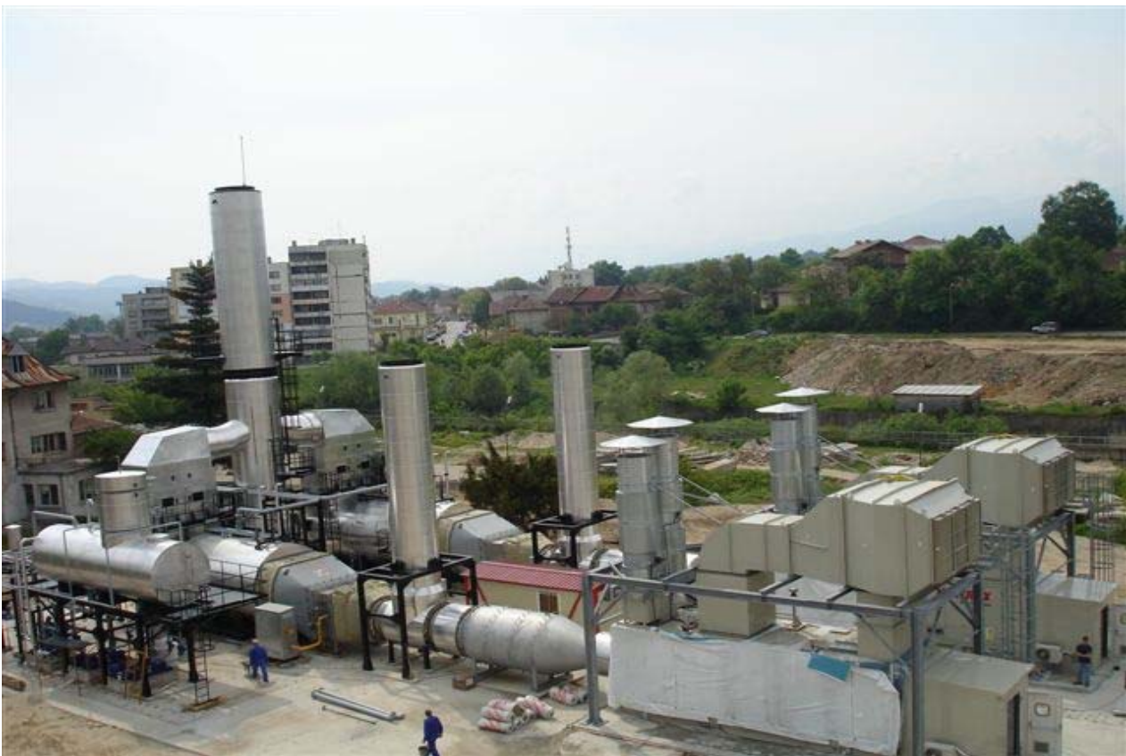
Fig.1.4.1 – Cogeneration installation at Kostenets HHI common view
