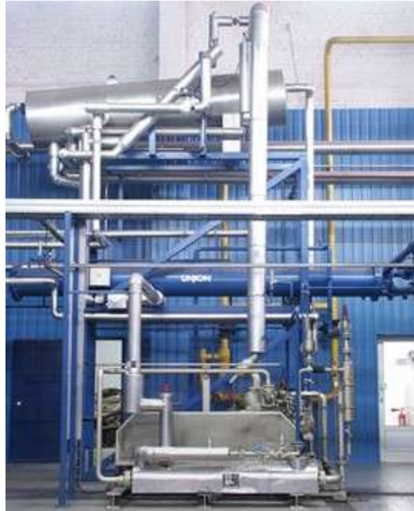
Fig. 2. Exterior of production systems of carbon dioxide of Union Engineering.
