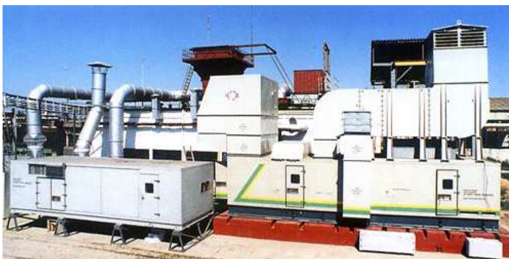
Fig. A 4-5. Gas turbine energy generation unit EG 6000
