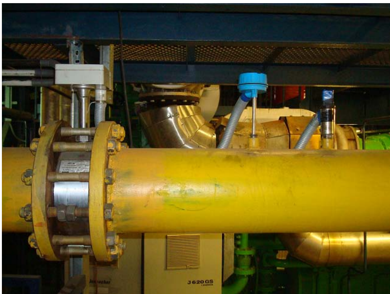
Figure 4: Sensors of flow, temperature and pressure at the CHP unit fuel methane pipeline
