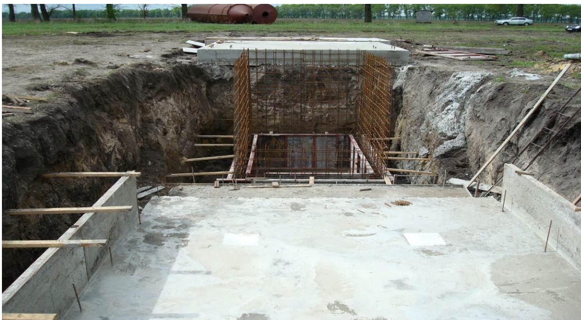
Picture 14. Building and assembly jobs on the farm construction site in Chernigiv oblast, Borzniansky region, v. Komarivka.
