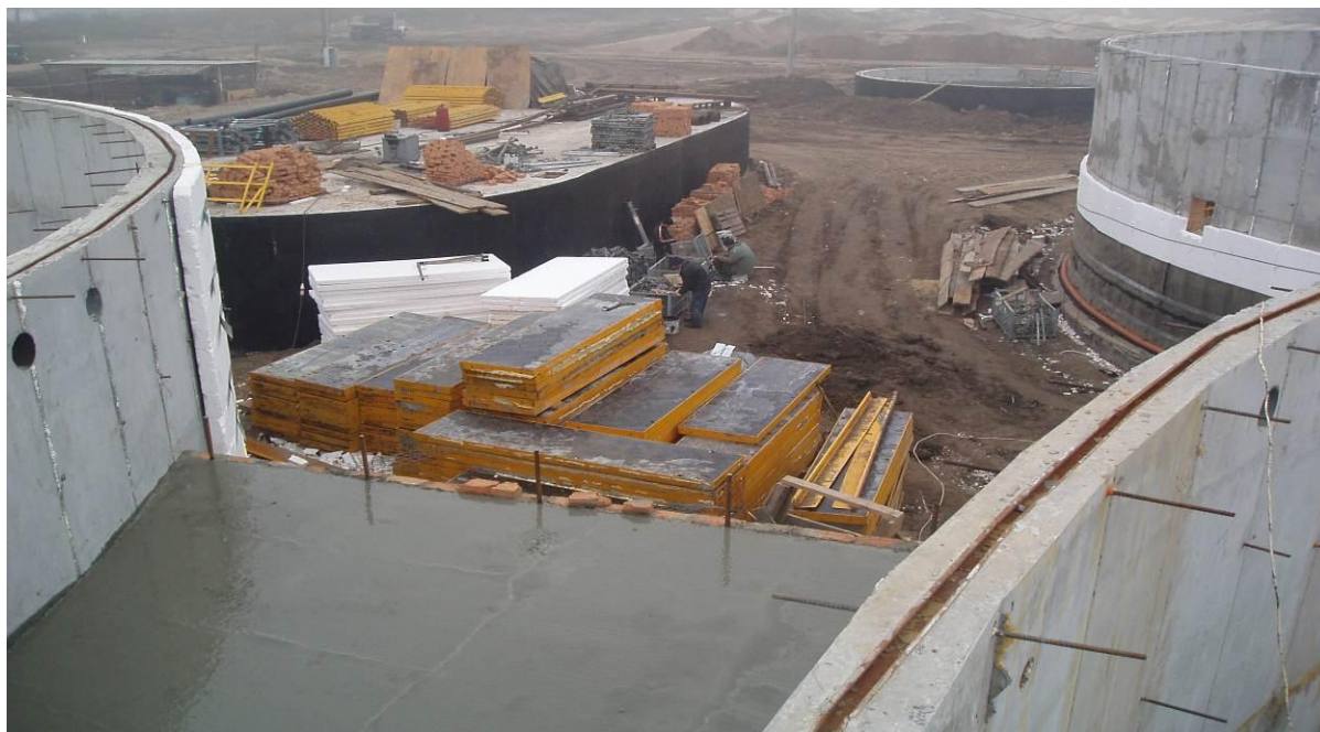
Picture 7. Construction of a biogas plant at the farm in Kyiv oblast, Zgurivsky region, v. Velyky Krupil.
