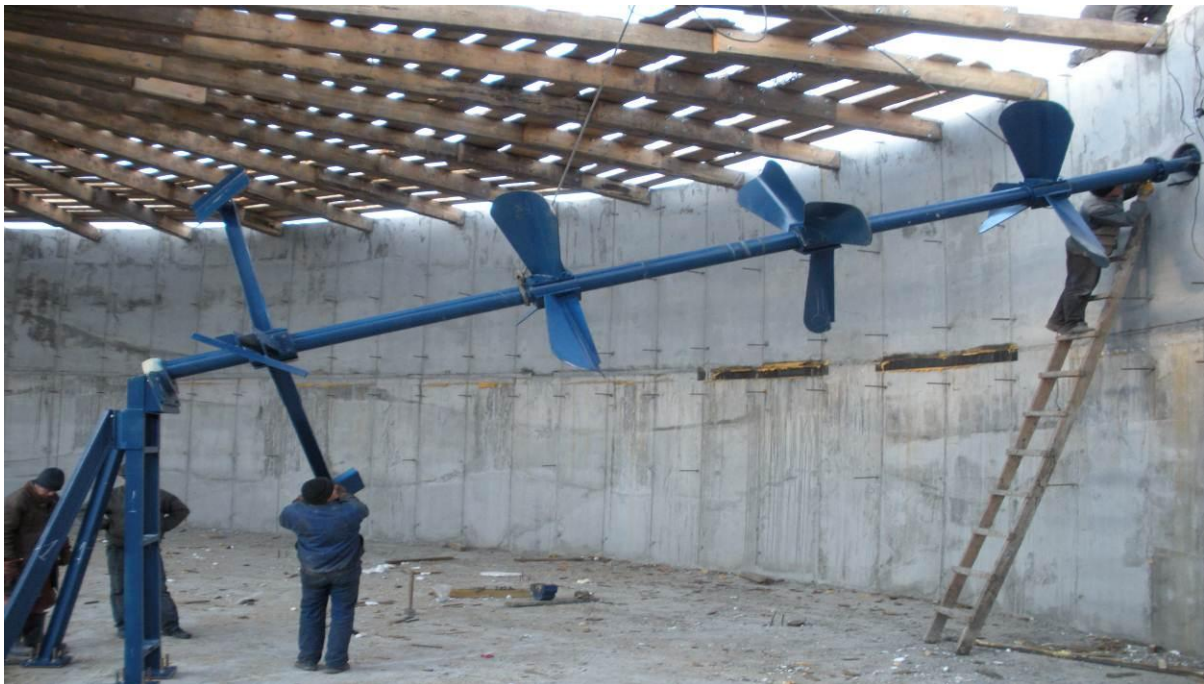
Picture 11. Equipment for mixing manure during their fermentation in a fermenter (construction site: Kyiv oblast, Zgurivsky region, v. Velyky Krupil).
