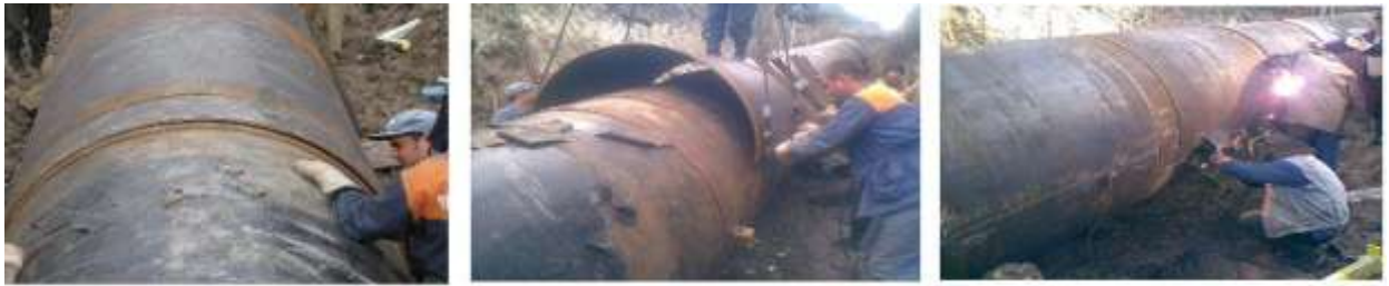
Figure 8: Application of two-layer sleeve – from left to right: adjustment of the rings and sleeve, assembling of the sleeve (rings on place), welding (a chain of several sleeves is shown which is covering multiple defects).
