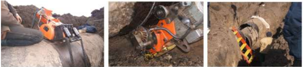
Figure 4: Cutting off the damaged pipeline section – still the predominant repair method in the beginning of 2000 th .
