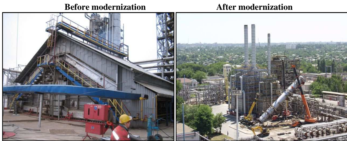
Fig. A.4.-3. Furnaces of the AVD unit before (on the left) and after modernization (on the right)
