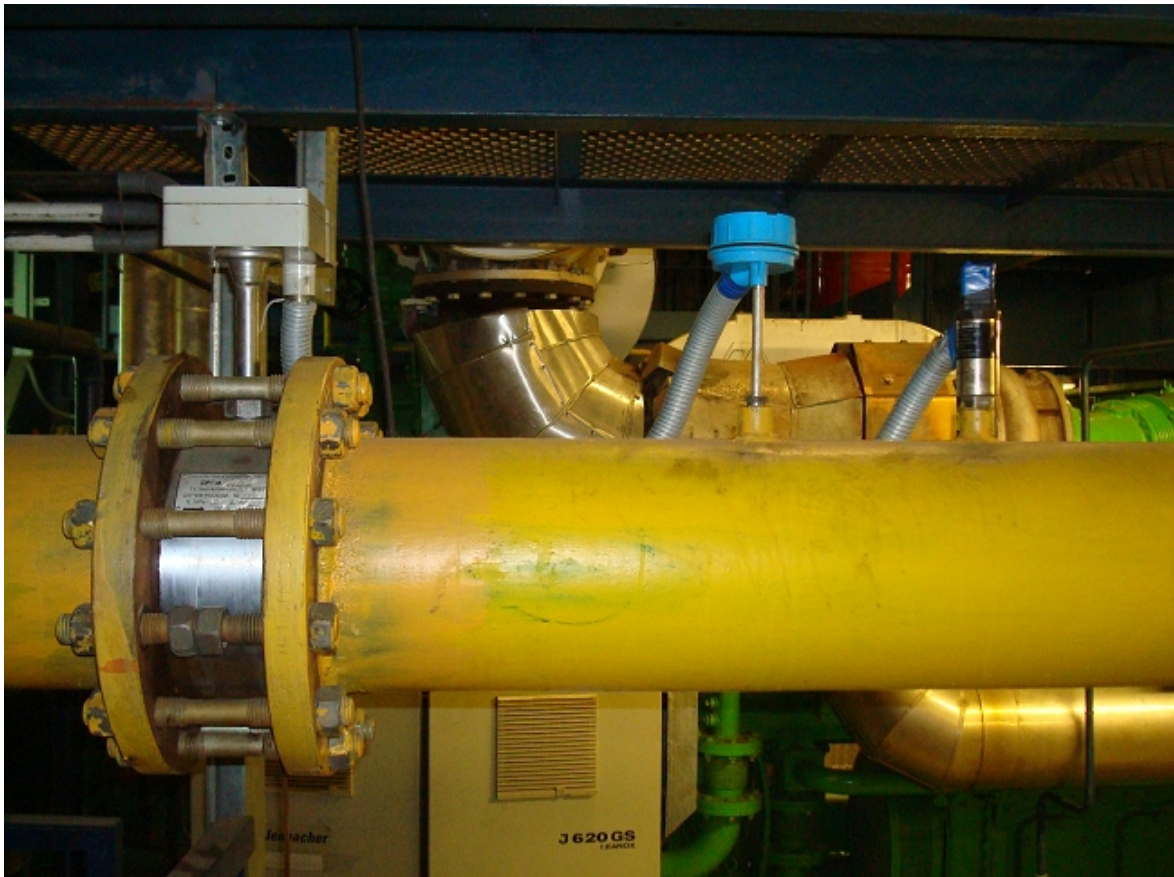
Figure 5: Gas flow meter DRG.M-10000 12 temperature sensor Metran 274-02 and pressure sensor Vegabar-14 of metering system for gas record BKT.M at fuel gas pipeline of CHP unit.
