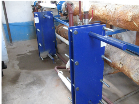
Fig. 1 New heat exchangers
