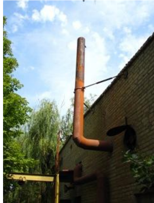
Fig. 5 Stand at degasification station releasing CMM into the atmosphere.
