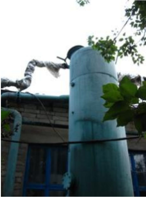
Fig. 4 Part of gas preparation station.
