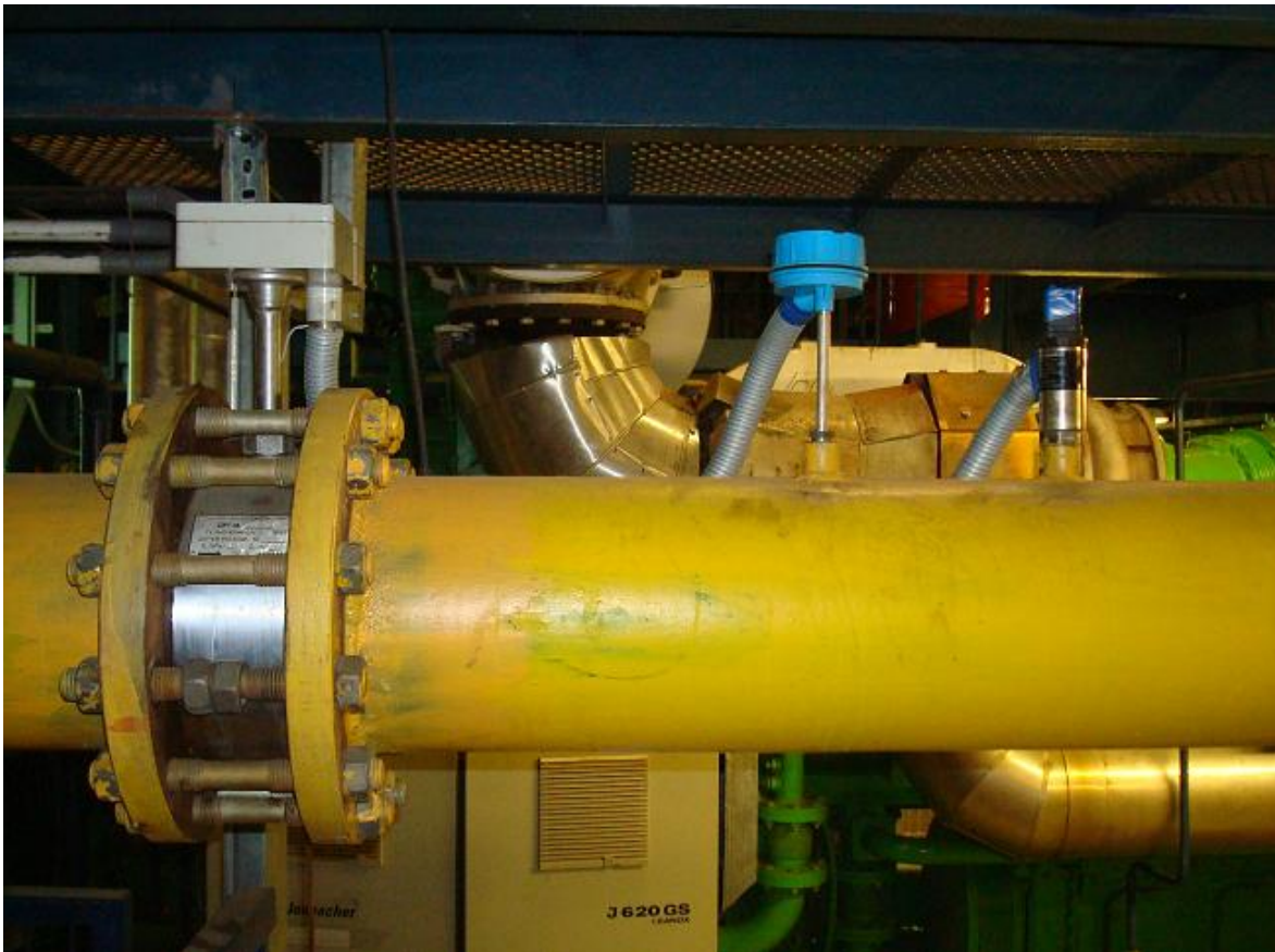
Figure 6: gas flow meter DRG.M-10000 11 , temperature sensor Metran 274-02 and pressure sensor Vegabar-14 of metering system for gas record BKT.M at fuel gas pipeline of CHP unit.
