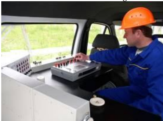
SS 110/10kV «Krystal». Transportable control laboratory TCL-110. Current transformers control 10kV without their dismantling. Post.
