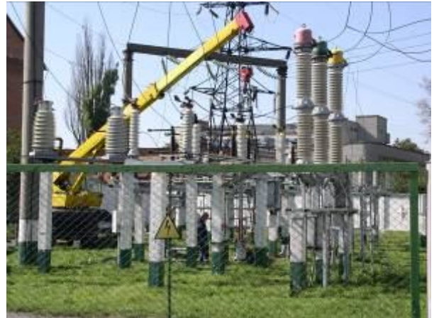
SS-110/10 kV «Tsentralna». VRU-110 kV . Replacement of the oily switch VMT-110 B for the gas-insulated switch 110 kV (Siemens production).
