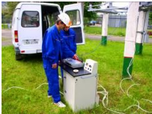
SS 110/10kV «Tsentralna». Transportable control laboratory TCL-110. Current transformers control 110kV without their dismantling.
