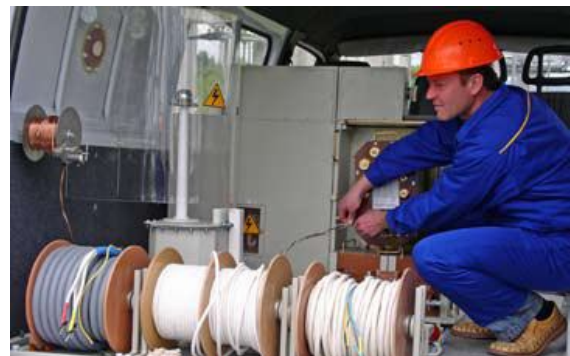
SS 110/10kV «Krystal». Transportable control laboratory TCL-110. Current transformers control 10kV without their dismantling. Prepaation of the measurement scheme.
