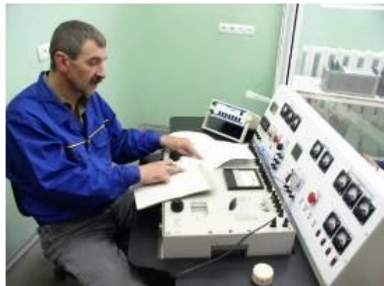
Relay protection service. Stationary control laboratory SCL-10 for the current and voltage transformers control. Voltage transformers control 10kV.
