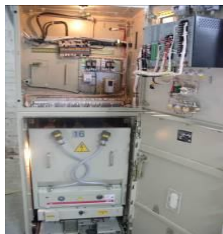
SS 110/10kV «Dubovo». Cell 10kV after the vacuum switch installation
