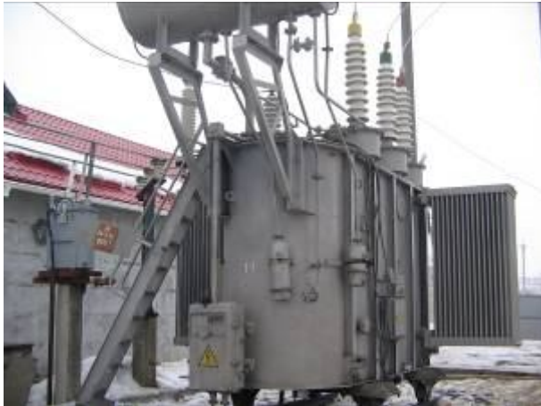
SS-110/10 kV «Krystal». Power transformer 6,3 MVA after installation.
