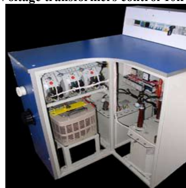
Stationary current transformers control device.
