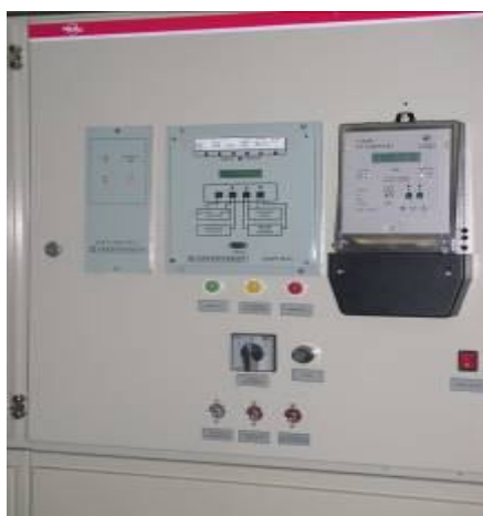
SS 110/10kV «Dubovo». Cell 10kV after the reconstruction
