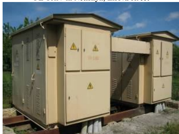
Double-transformer substation 10/0,4kV Stara Ushytsya.
