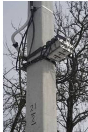
Sectional switch 0.4 kV, Netishyn.
