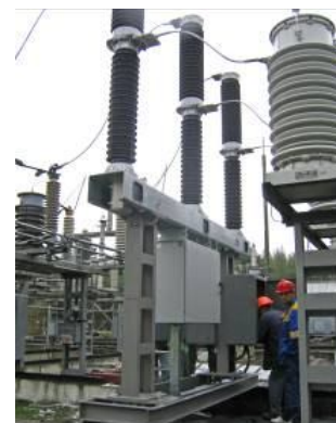
SS-110/10 kV «Tsentralna». Gase-insulated switch 110 kV(Siemens production)
