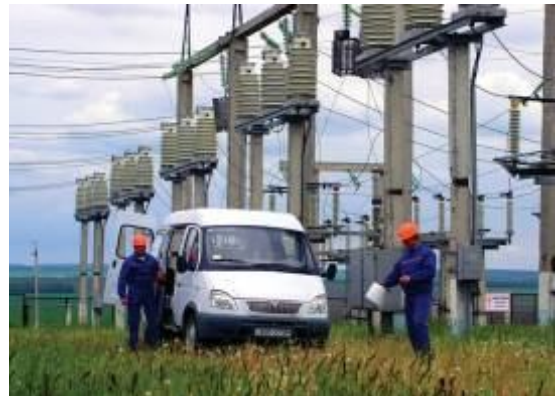
SS 110/35/10kV «Yarmolentsi». Transportable control laboratory TCL-110. Current transformers control 110kV without their dismantling.
