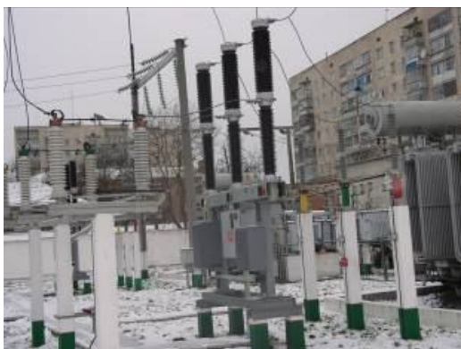
SS-110/10 kV «Tsentralna». VRU-110 kV after the reconstruction.
