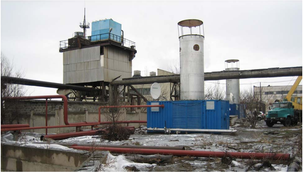
Figure-4 Flare 3 and Flare 4 – Komsomolets Donbassa Coal Mine, Air Shaft Nr.3
