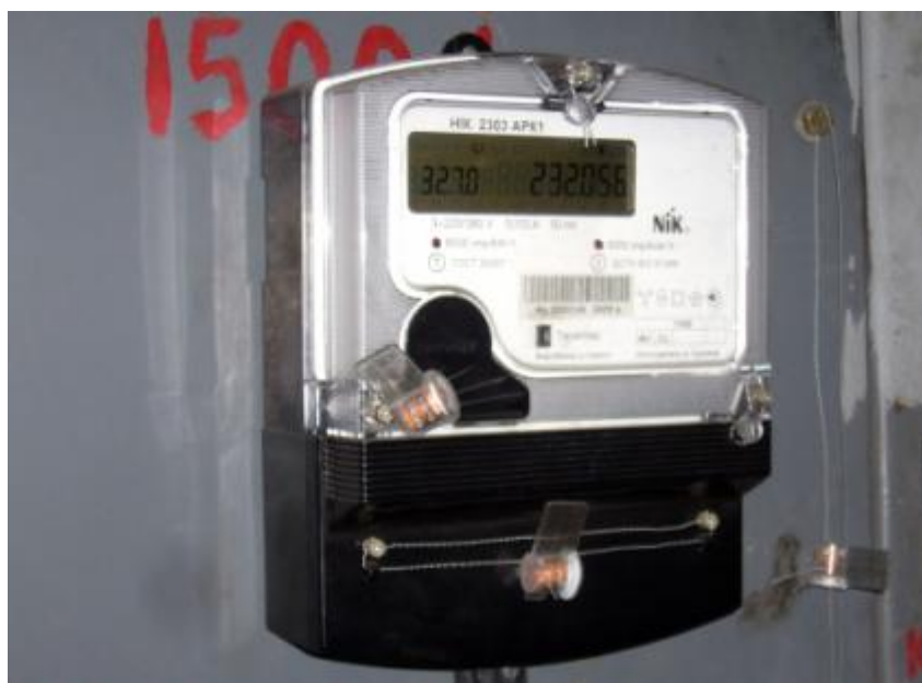
Figure 2 Electricity meter “НИК 2303АПК1”
