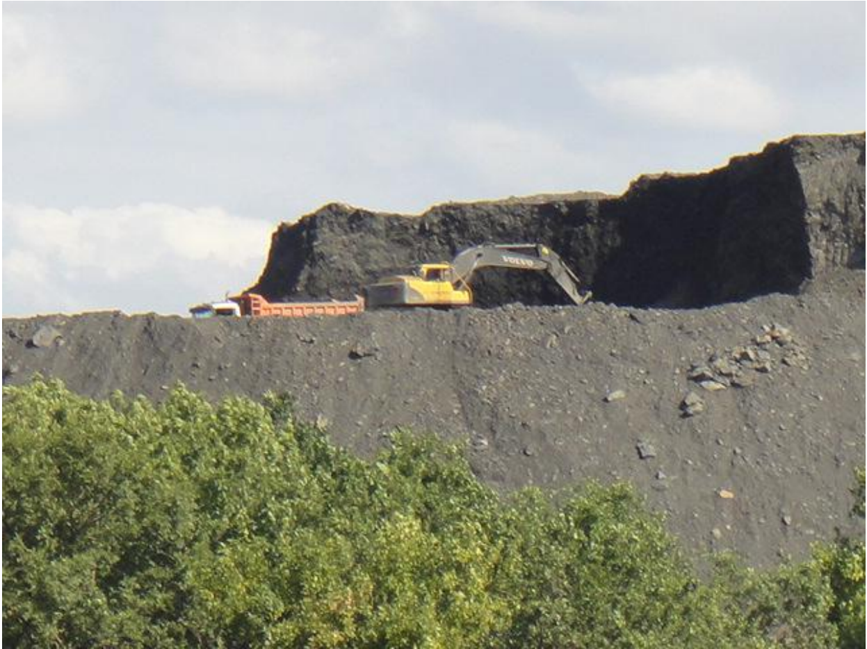
Figure 3 - The exterior of the waste heap#1 at Vahrusheva mine under dismantling stage
