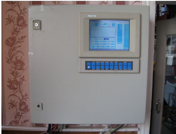
Fig. 4 automatic systems “ПОТОК-ДН-03”
