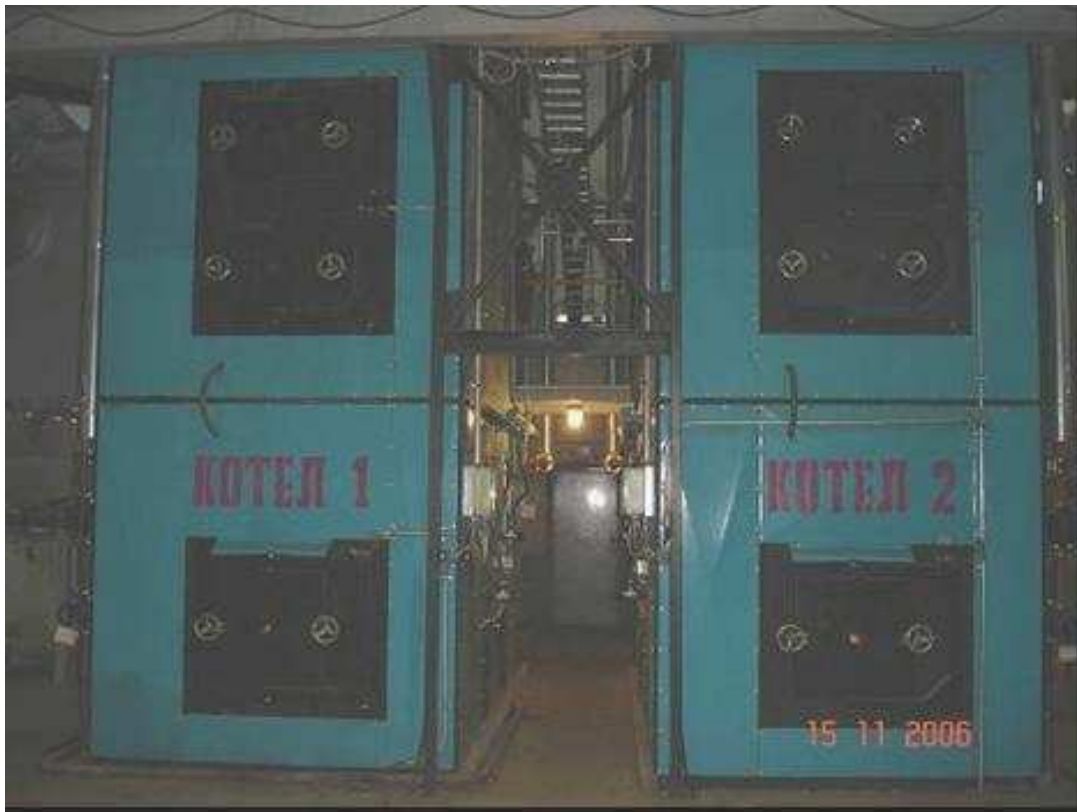
Fig. A.4-7. Utilizing boilers “Polytechnik”
