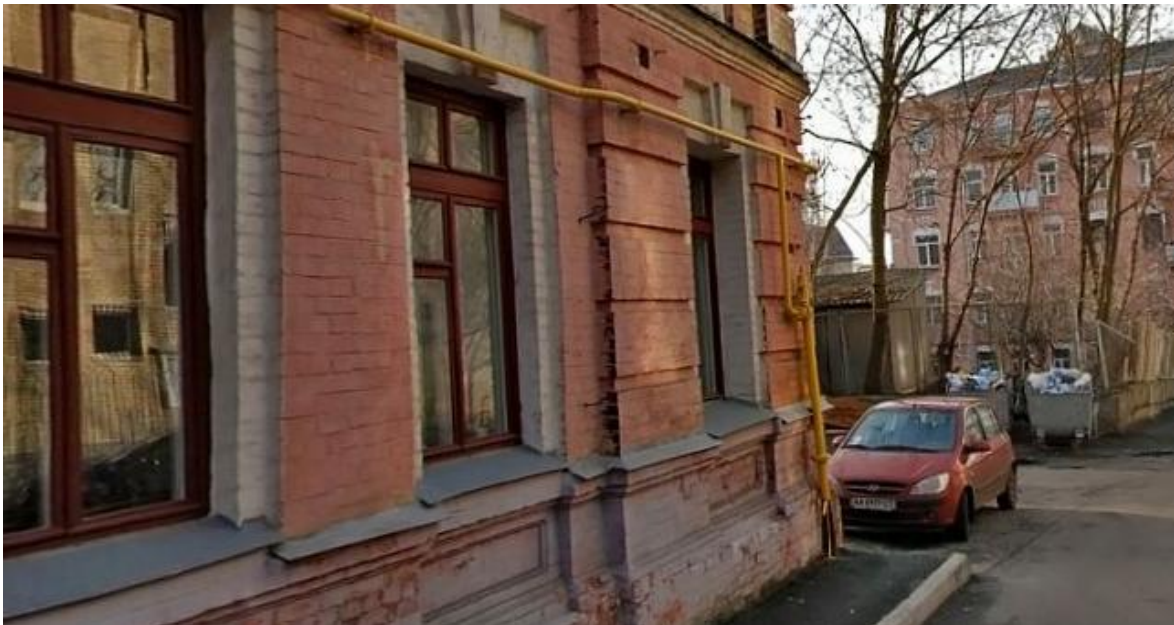
Figure 2. A low-pressure gas pipeline built within the project “Reduction of greenhouse gases emissions by gasification of Kyiv city” (Kyiv city)
