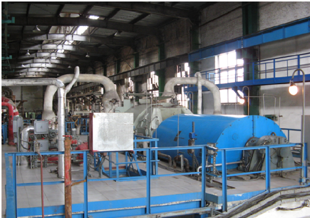
Figure 6. Location of the PT-12 turbine in the block of JSC «YCP» CHP plant.
