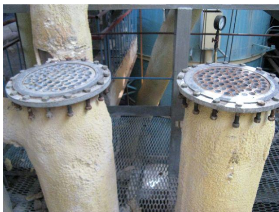
Figure 7: Heat exchange equipment surface 15
