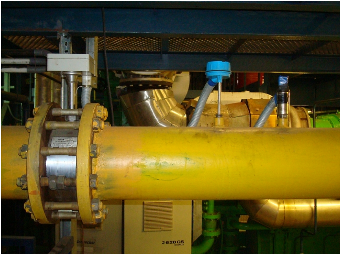
Figure 5: Gas flow meter DRG.M-10000 12 temperature sensor Metran 274-02 and pressure sensor Vegabar-14 of metering system for gas record BKT.M at fuel gas pipeline of SU CHP unit.
