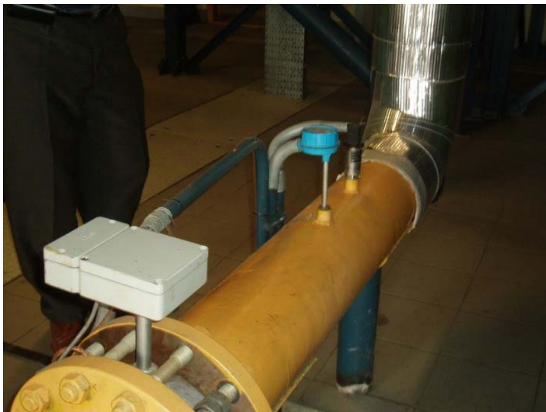
Figure 4: Sensors of flow, temperature and pressure at the CHP unit fuel methane pipeline
