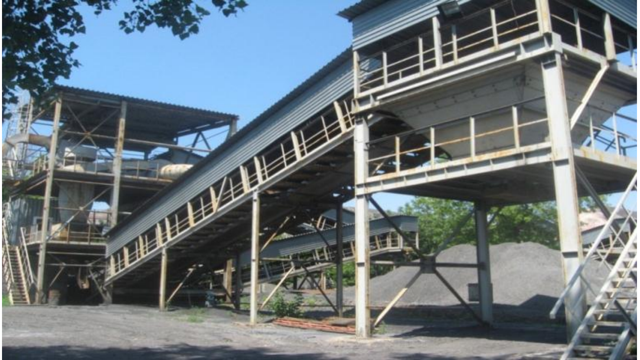
Figure 4: View of beneficiation plant for waste heap processing that is being dismantled in the project
