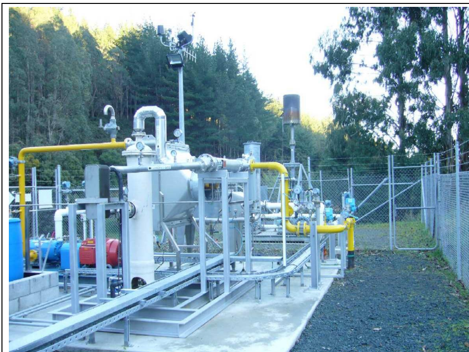
Landfill gas treatment plant, Flare in background
