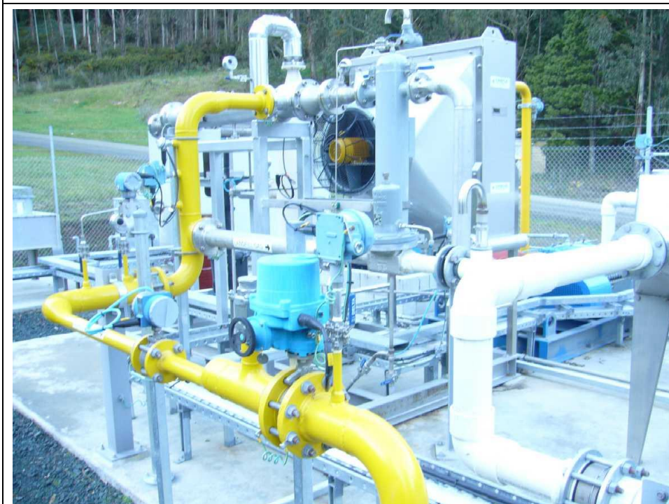
Landfill gas treatment plant. Incoming gas is compressed, filtered, and chilled before sent to the hospital boiler via an underground pipeline. The gas is typically 55% methane and 45% carbon dioxide. Faults in the landfill gas collection system occasionally allow air ingress lowering this ratio. Such faults are monitored by the NCC and remedied quickly.
