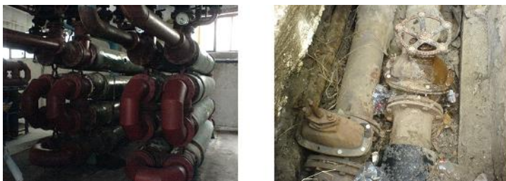
Figure 2: Heat exchanger and secondary district heating network pipes
