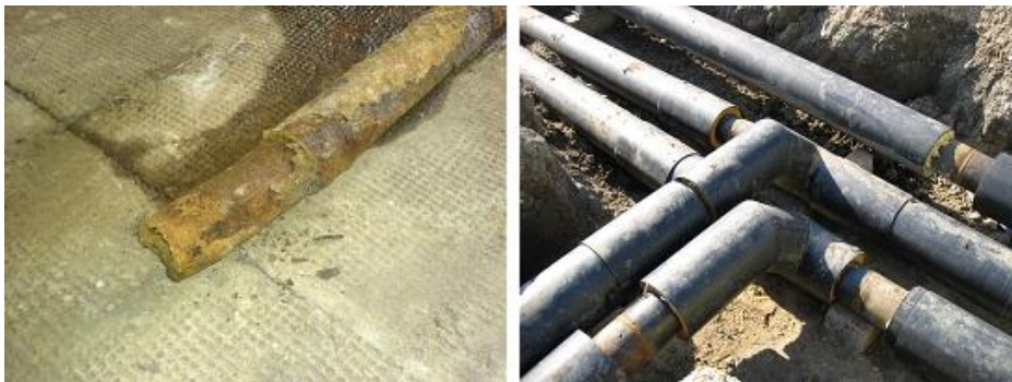
Figure 6: District heating pipes [old, new]
