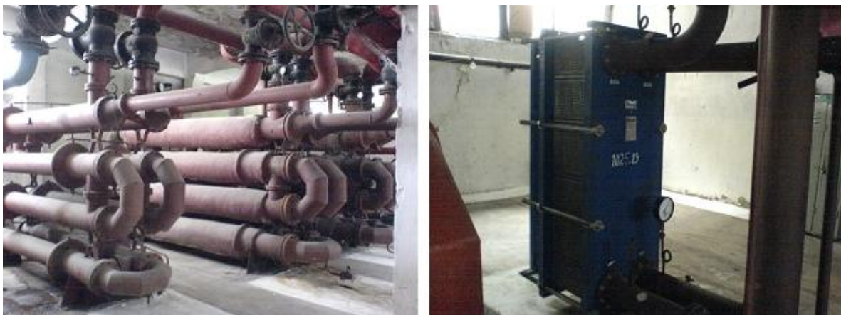
Figure 7: Heat exchangers [old, new]
