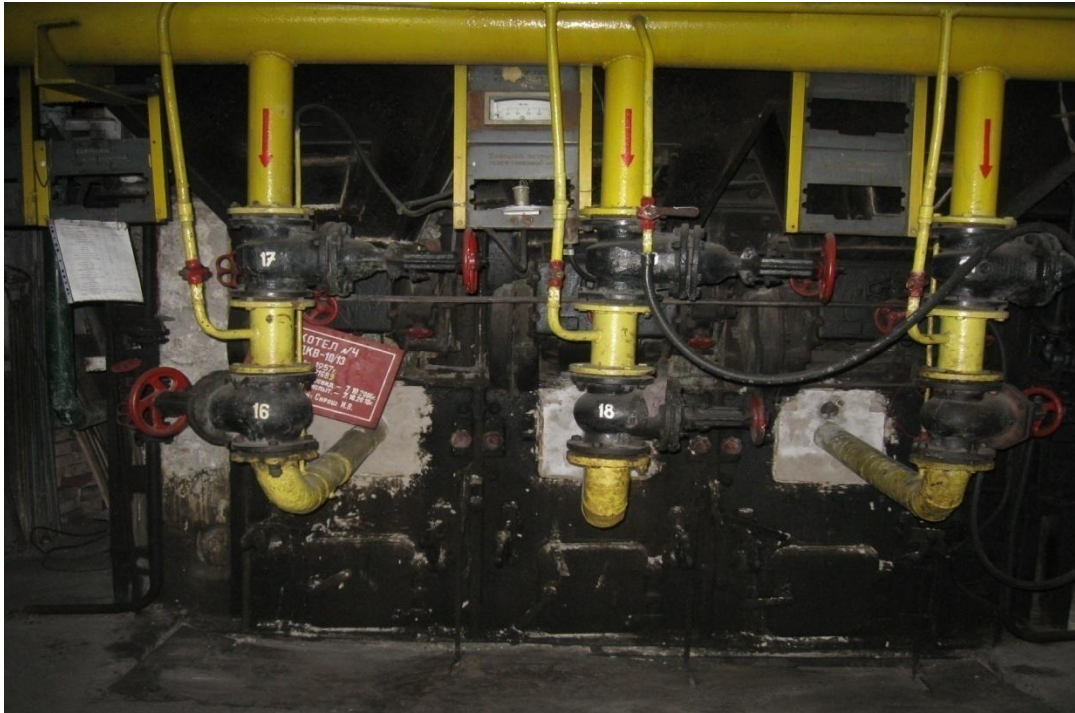
Figure 5. Modernized boiler DKVr-10/13
