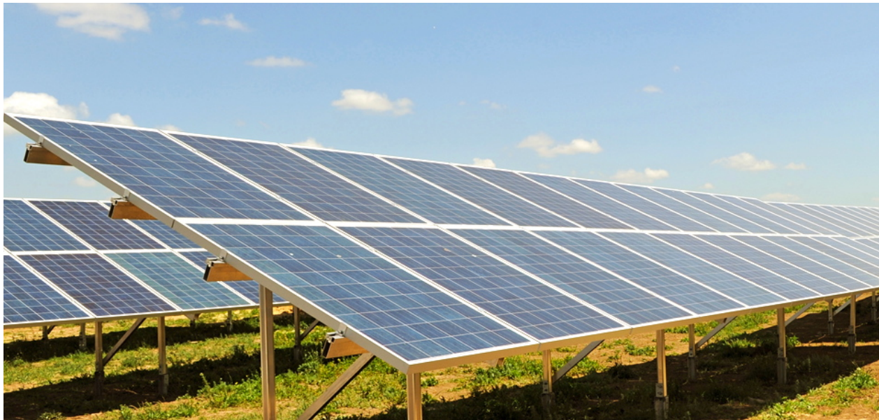
Figure 4. Photovoltaic panels installed.
