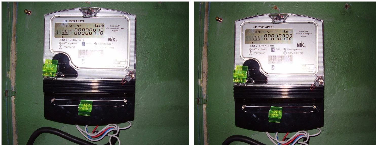
Figure 3 Electricity meter “HIK 2303APT2T”
