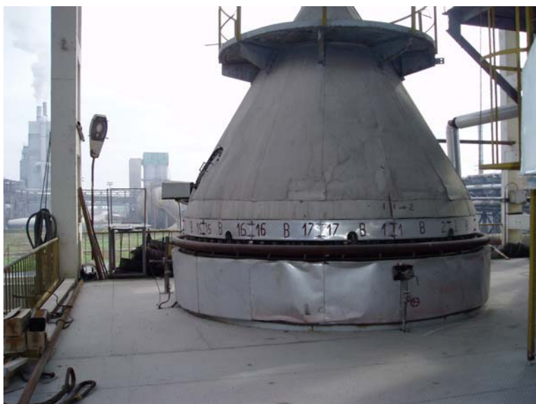
Figure 6 Foto of one of the four reactors (NH 3 burners)
