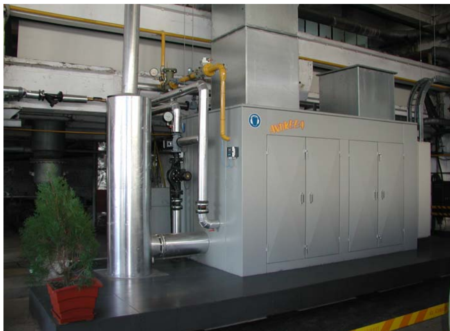
Figure 4 ANDREEA, the new cogeneration installation in operation in Târgoviște since October 2003
