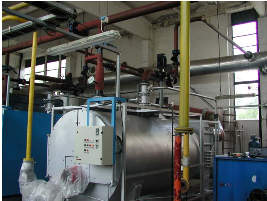
Figure 3 New heat only boiler during its installation last year in Sibiu
